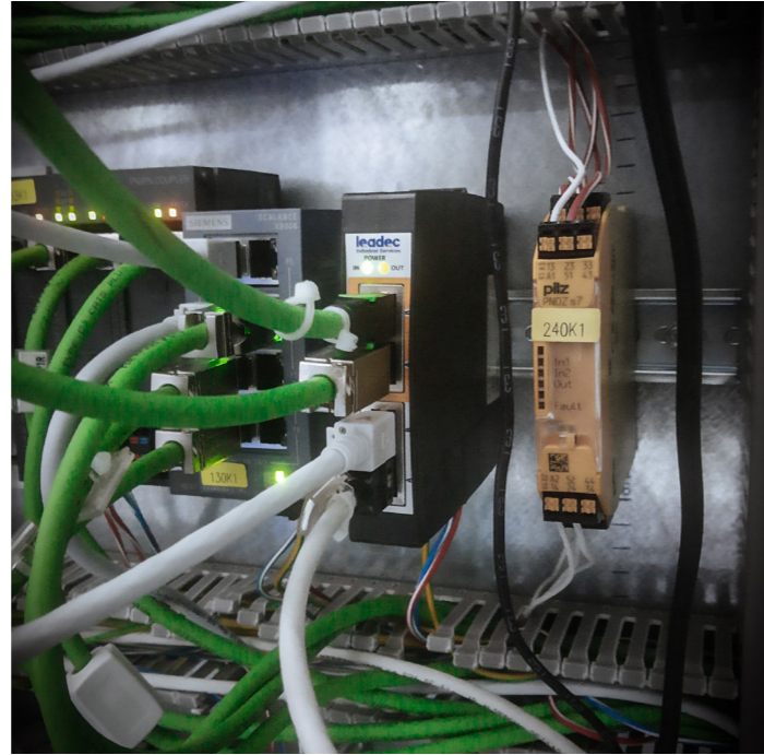
netMIRROR in operation at a Leadec-supervised plant
